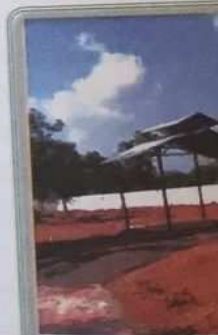
Picture 8: Incomplete work
